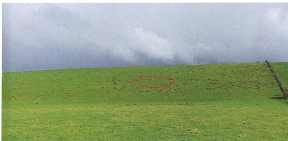
Figure A 2: Downstream face of the eastern embankment - note "wet patch" in middle of photo
