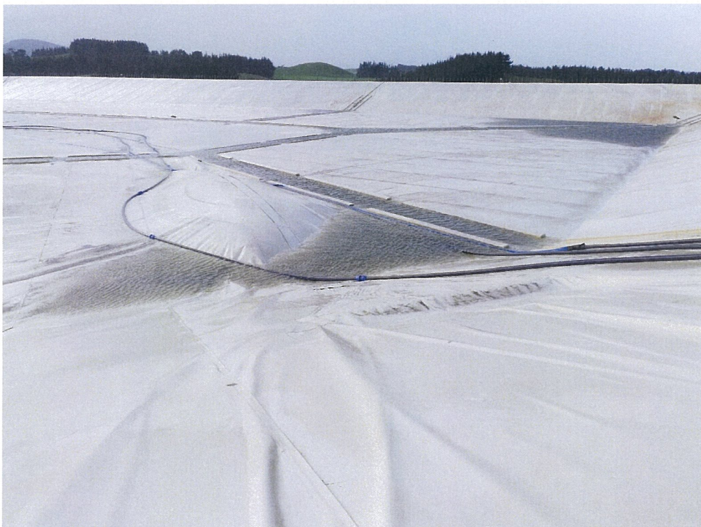
Figure A 1: Reservoir cover noting depression under the cover near the middle of the photo is the location of the inlet
