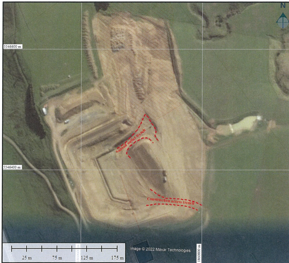
Figure 3.1: Deep trenches cut through eastern fill embankment during construction (photo dated 23 August 2012, taken from Google Earth, overlaid on as-built drawing sheet 2)
