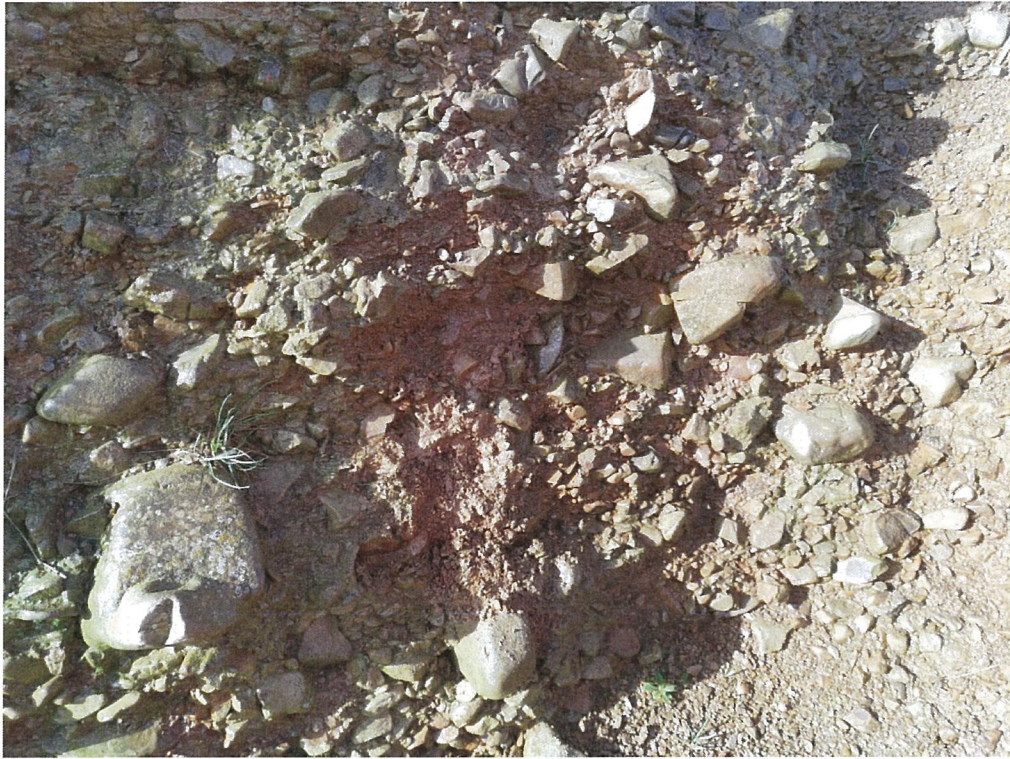
Figure A 8: Natural materials (silty gravel) exposed in cut alongside access track to reservoir
