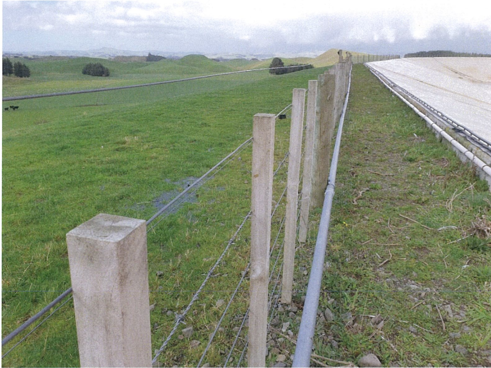
Figure A 6: Water ponding on crest of the eastern embankment
