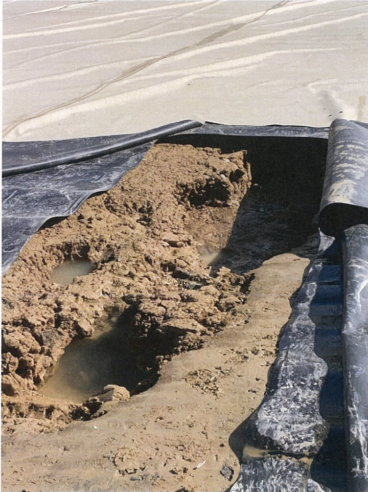
Figure 3.4: Damage below liner near top of slope during 2021 leakage incident
