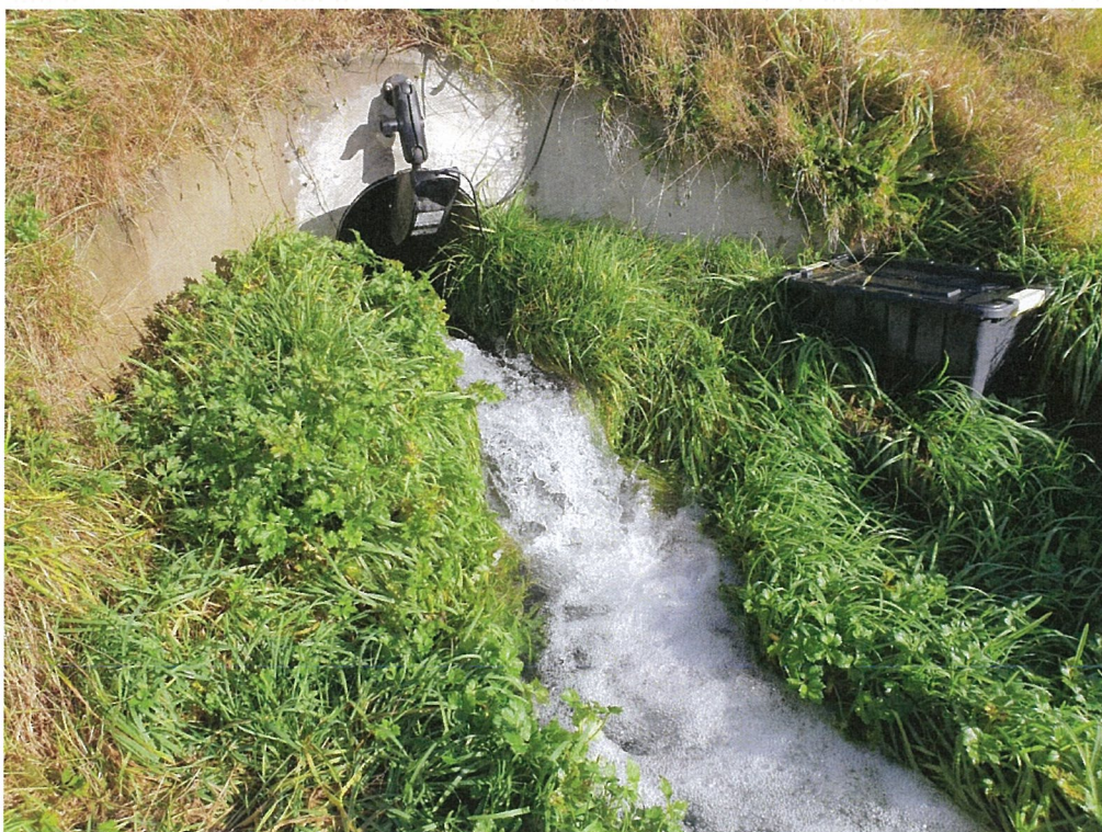
Figure A 7: Seepage flow at subsoil drain outlet to stream
