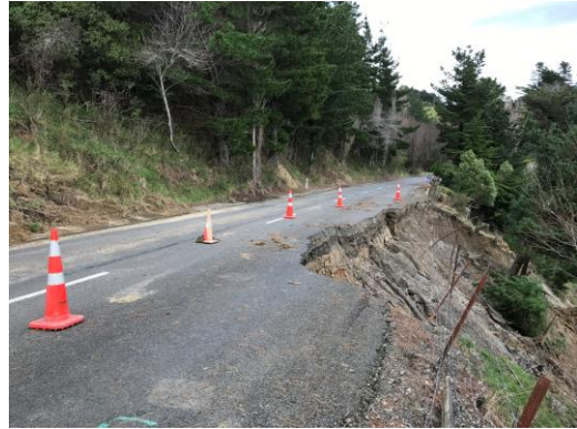
Road slumped into gully – Route 52
