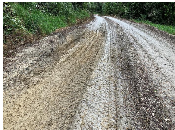
Damage to Unsealed Road through Logging Activity
